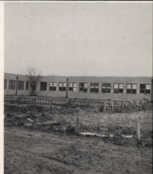
Work began on the new addition to the main building. This will give additional classrooms and a new office for the principal.
