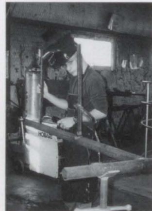
Left: Stabilizing a structure, Joey Quinney welds pipes together. Joey says that his favorite part about working on the steel structure was "not having to do worksheets like the rest of my class."
