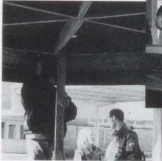
Ashlee Huffman and Chris Duke talk over what needs to be done next on the gazebo, while Tony Rodriguez works inside the gazebo.
