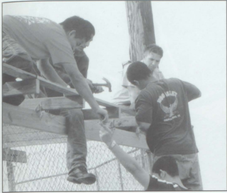
Juan Ayala, Nehemiah Juarez, Alex Nieto, and Justin Barefield work hard and fast building a roof on the dugouts at the baseball field.
