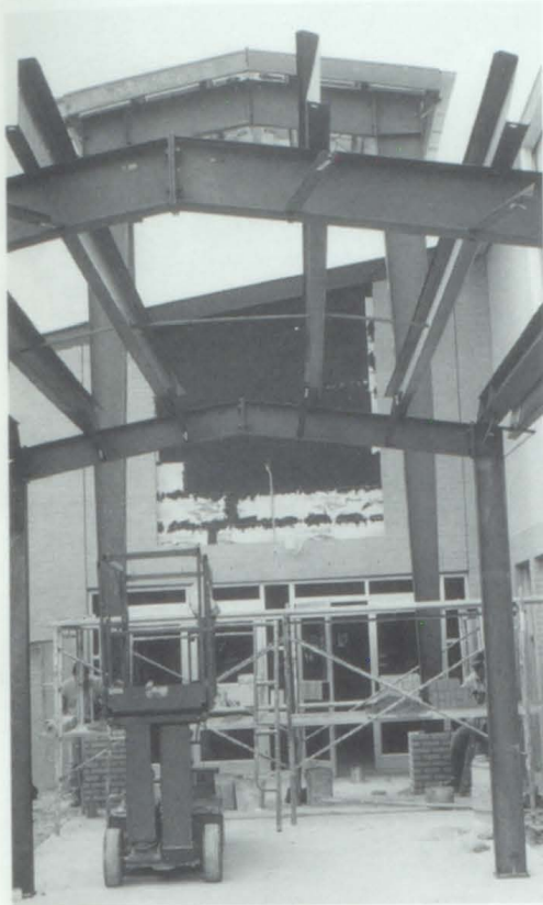
A grand new entrance shows how the construction at Central Elementary is off to a great start.
