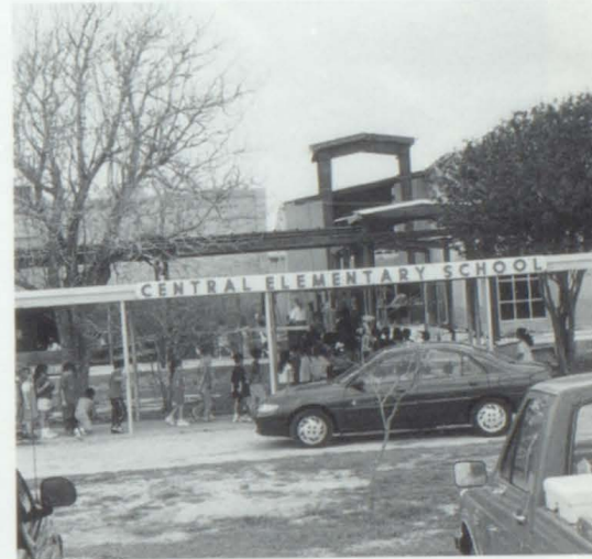
Each day, students watch the progress of the construction as they attend class and as they walk to the cafeteria for lunch.
